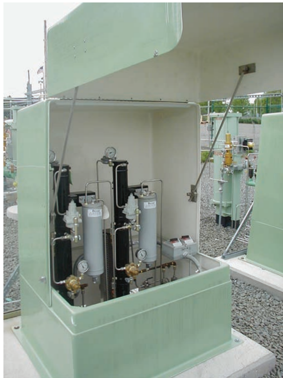
Figure 4 - Below Ground Regulator with Fiberglass Cabinet
