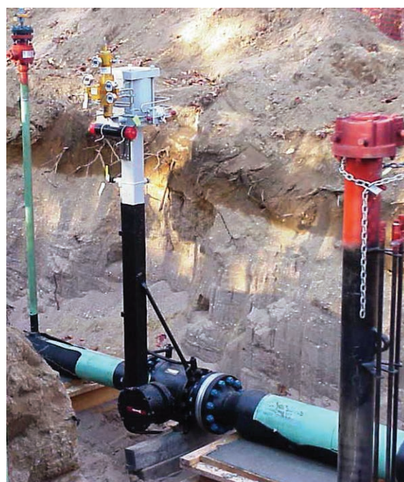
Figure 2 – Below Ground Ball Valve Regulator combined with Control Valve Silencer
